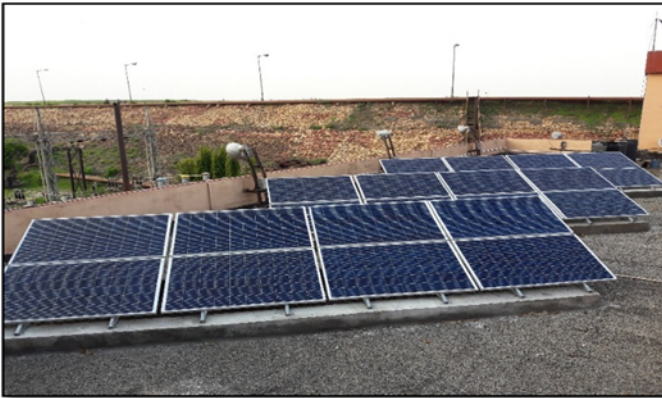
Solar PV Plant in Ash Pond.
