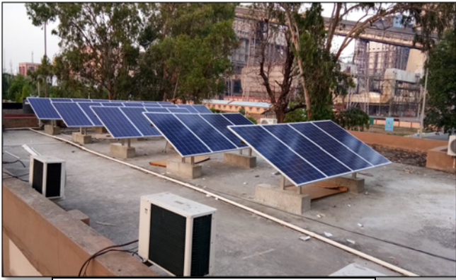
Solar PV Plant in Canteen.
